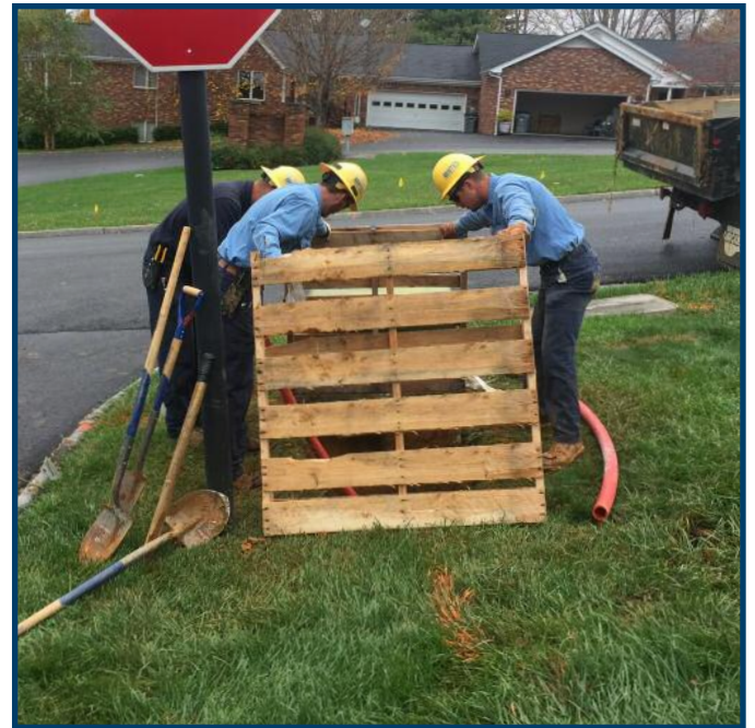
Once the boring work is complete, BTES crews install the new cable and make the necessary connections.
