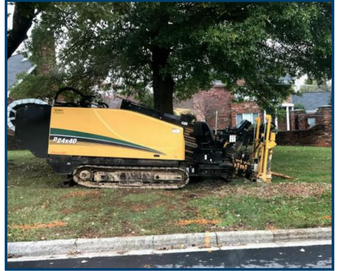
As crews work to replace underground facilities, customers will see directional boring equipment similar to what is pictured above.
