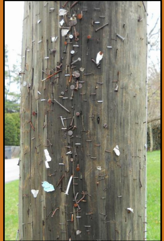
Photo of a pole in the BTES service area. Nails and staples pose a major concern for linemen.
