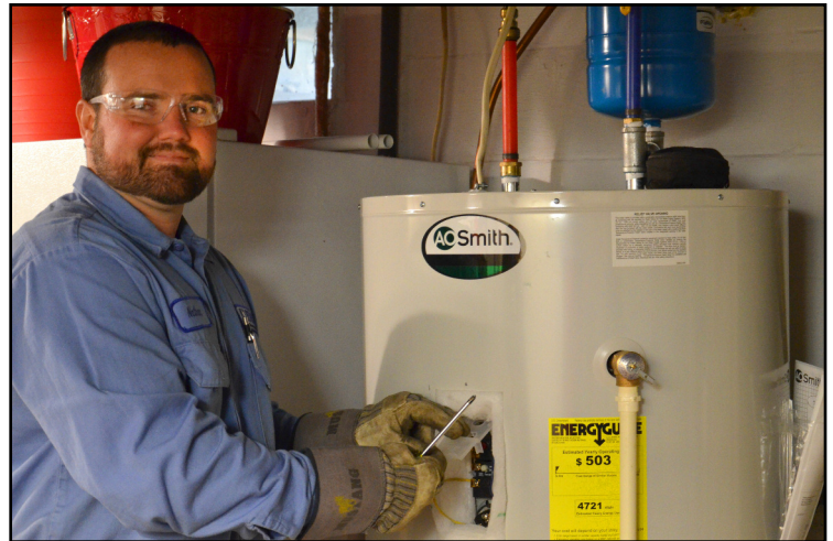
Nathan Meade, working foreman of meter and substations, installs a new load-management switch on a water heater.
